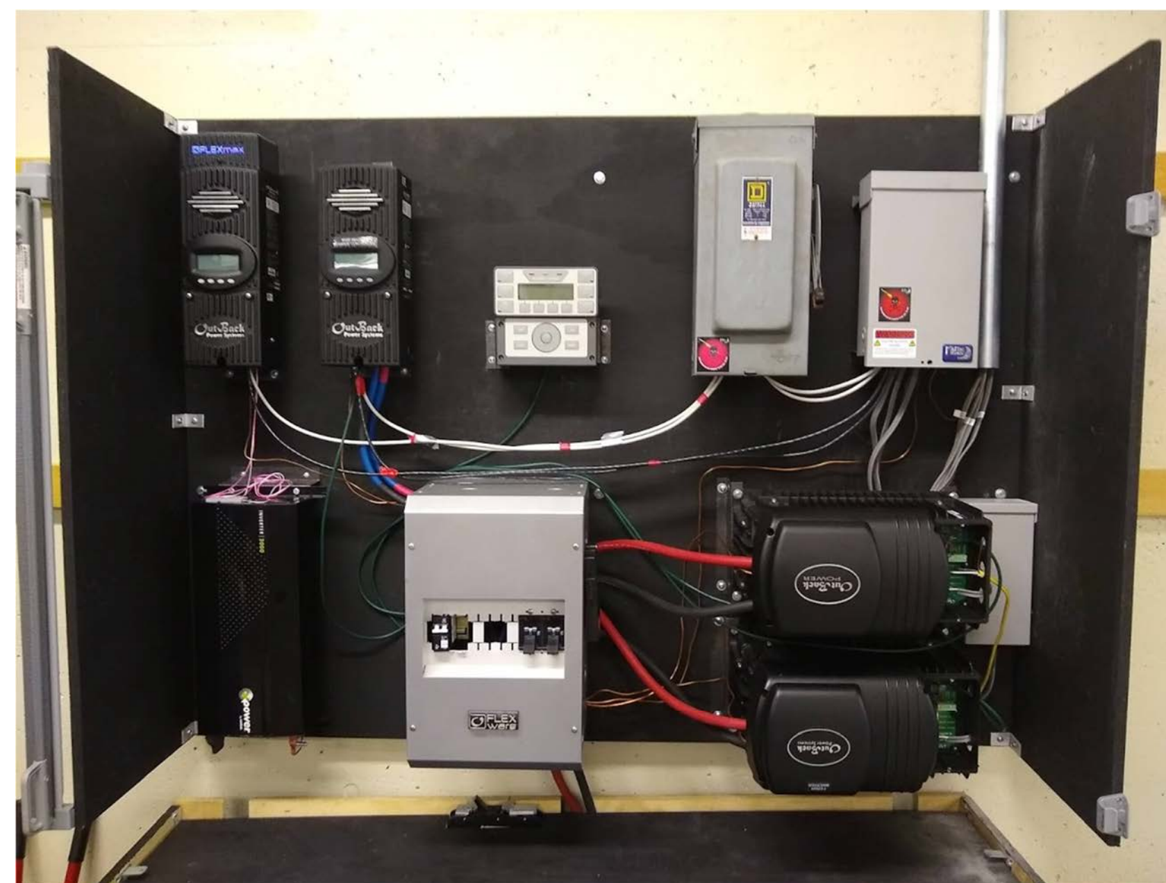
Figure 3: the Solar Lab Equipment Panel wired in spring 2021
